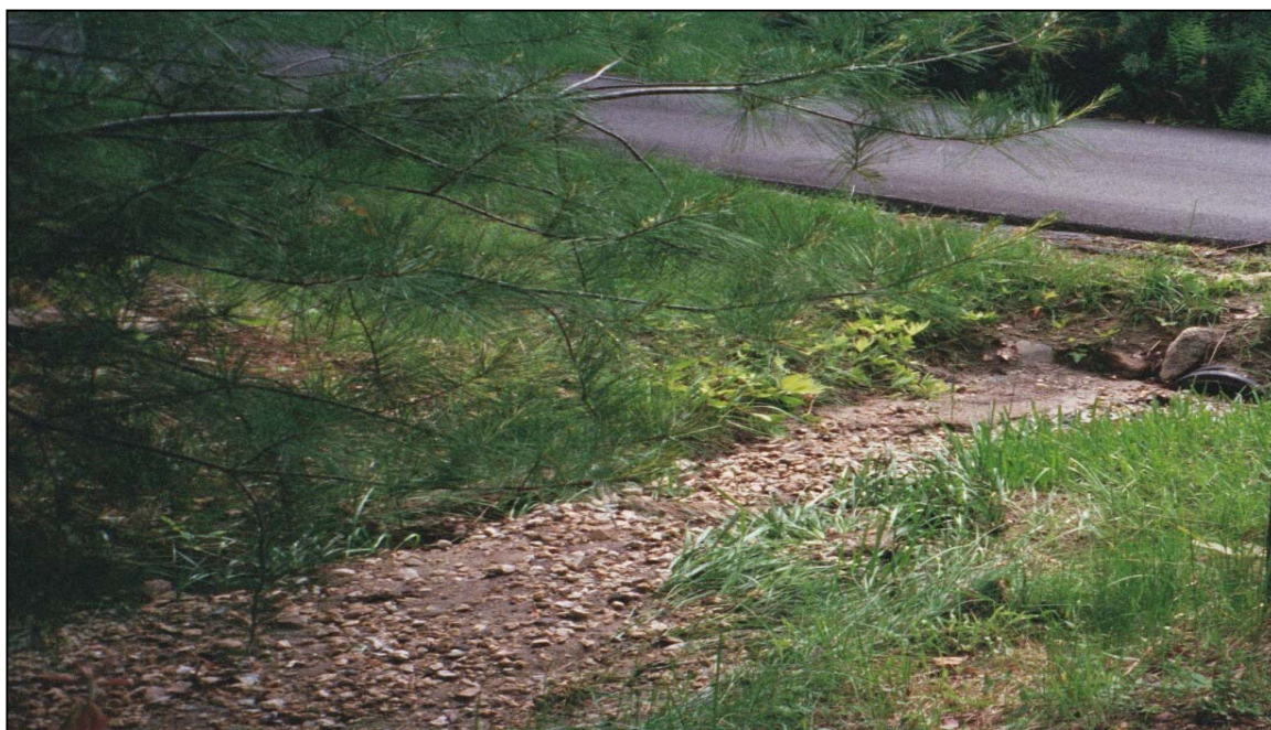
Figure 3-15. Wildwood Lane Clogged Driveway Culvert
