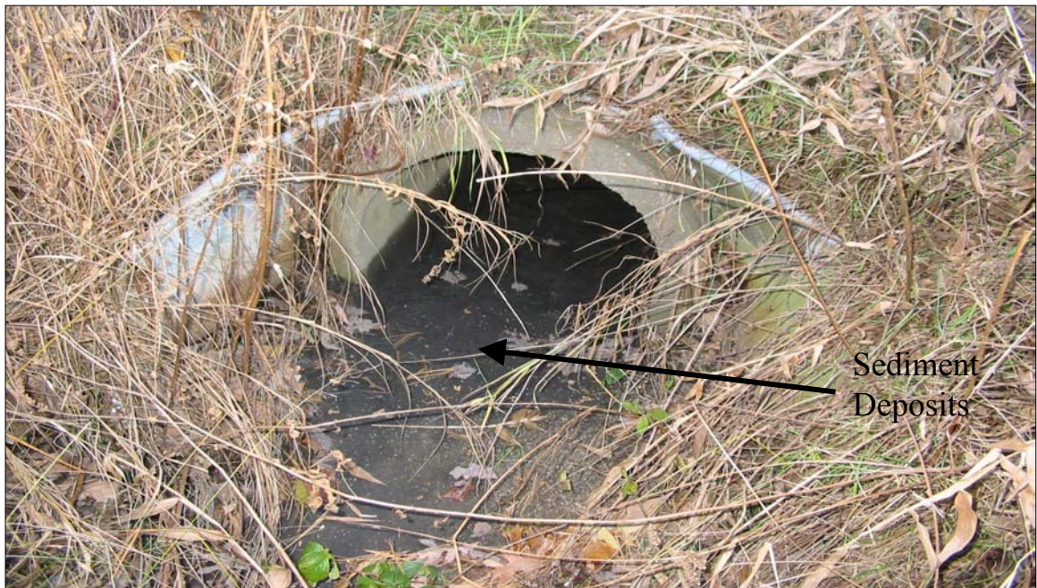
Figure 3-3. Route 101A 24” Discharge Upgradient of the SPB Outlet Wetland (Note heavy sediment deposits at pipe bottom)
