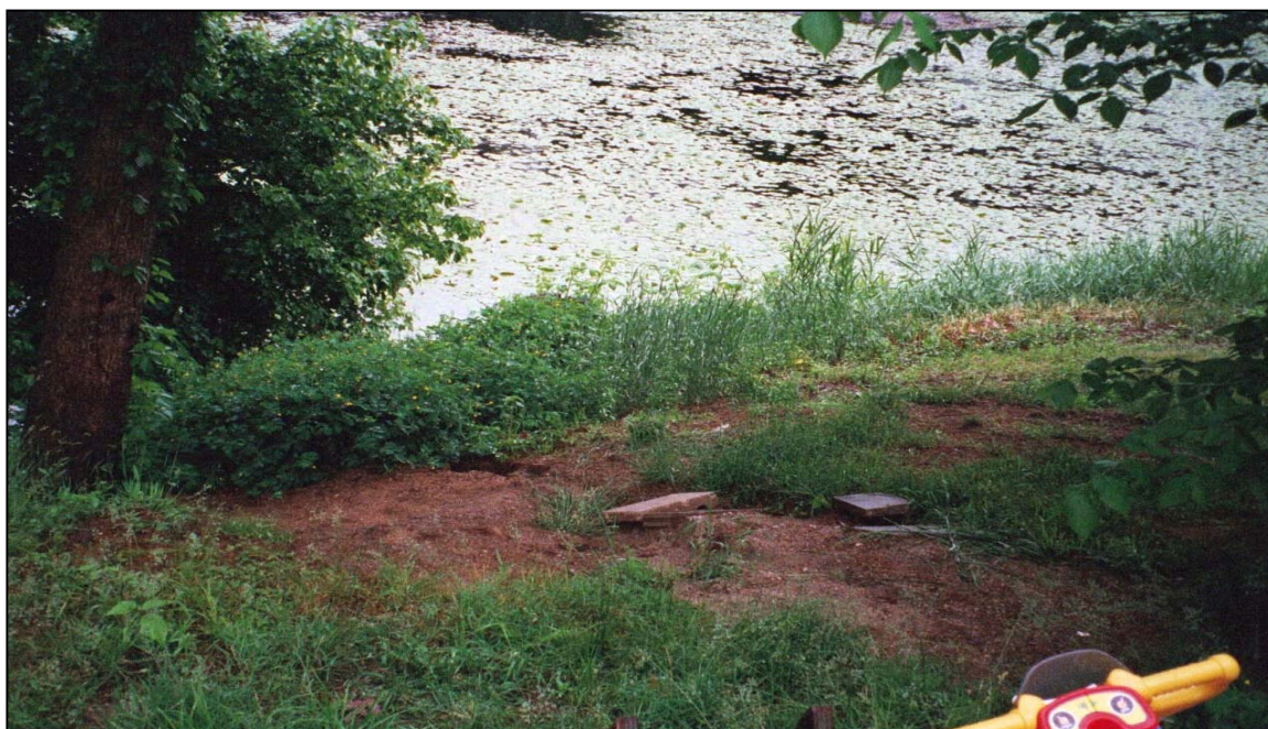
Figure 3-13. Willow Road Drainage Discharges into Stump Pond (Steep unstable bank is being eroded)
