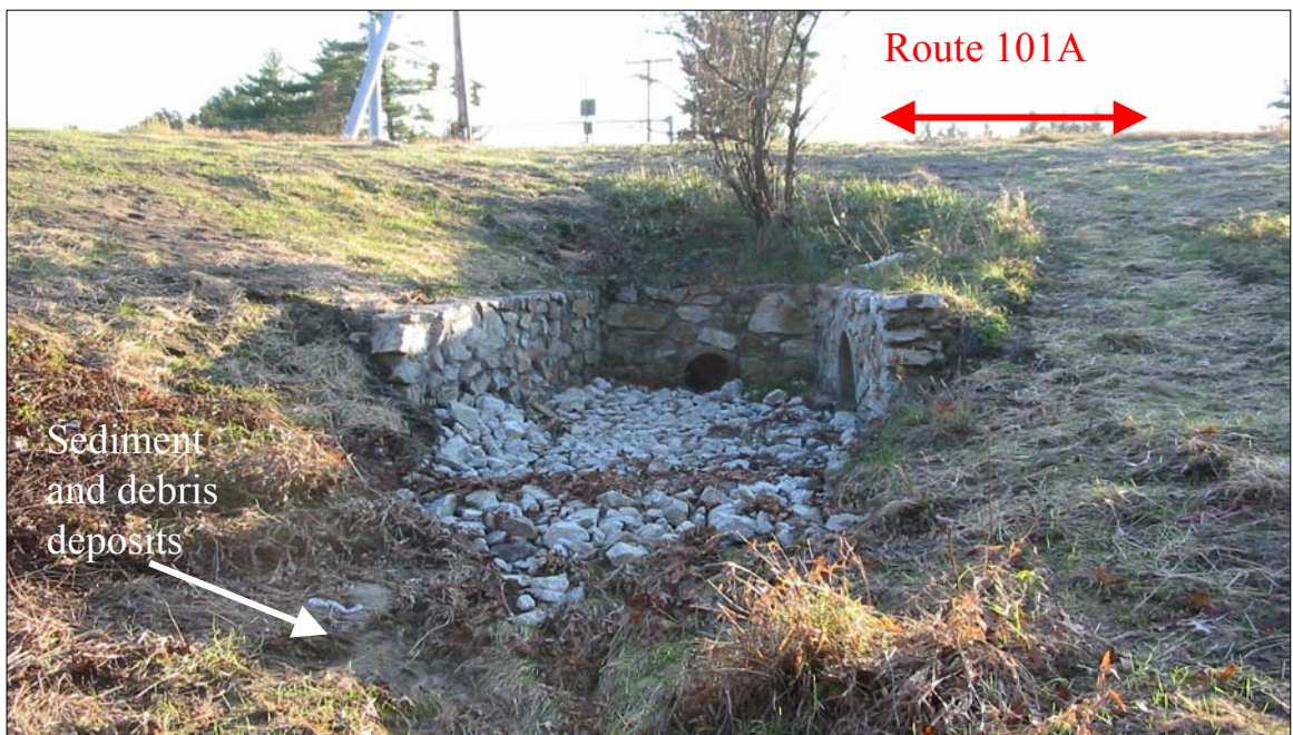
Figure 3-7. Route 101A Discharge to Stump Pond Facing Road
