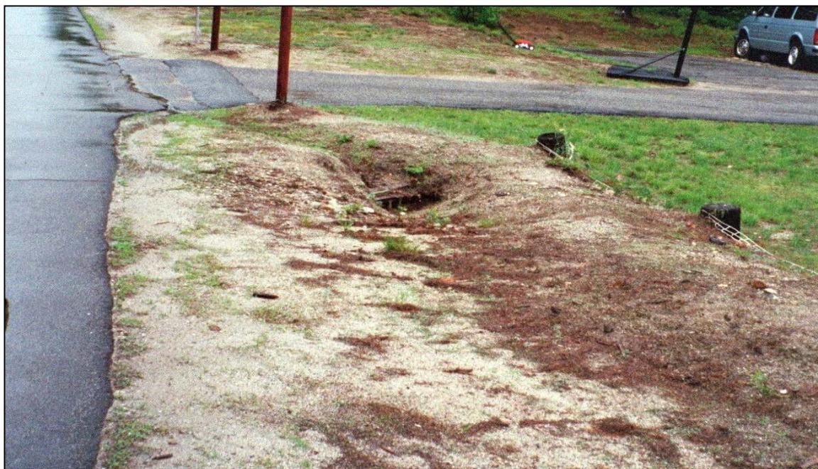
Figures 3-12. Clogged Catch Basin on Willow Road
