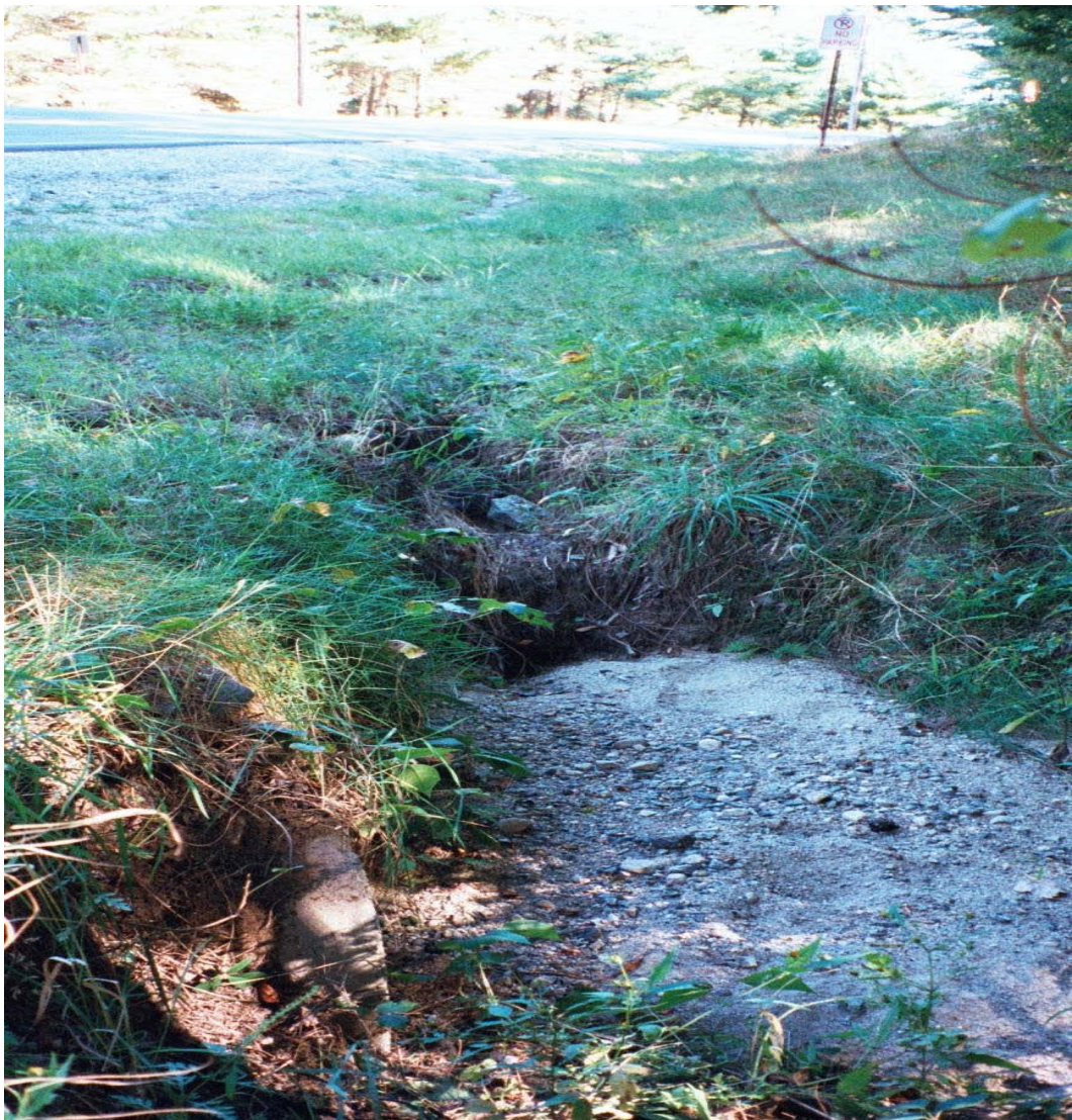
Figure 2-18. A large sediment delta observed before the 18'' culvert beneath Route 122.
