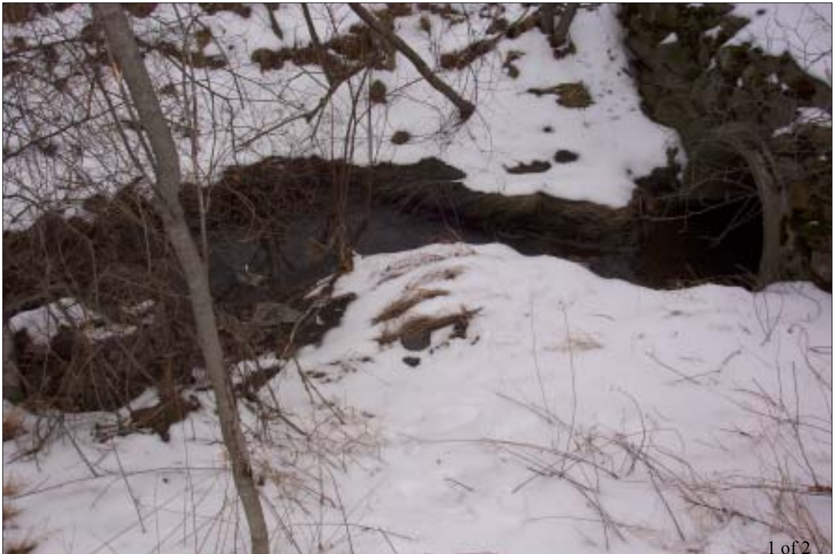
View of Drainage Outlet – High velocity flows has caused scouring of ditch
