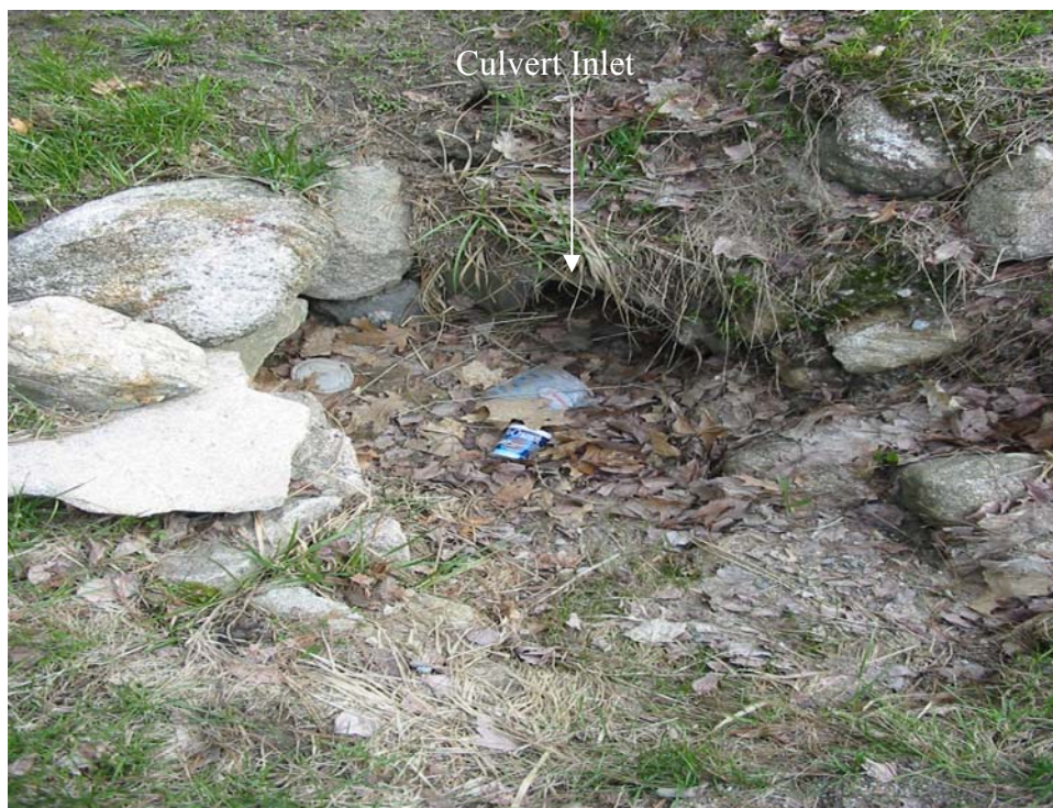
Figure 4-8 Sediment & Debris Collected in Inlet Side of Culvert
