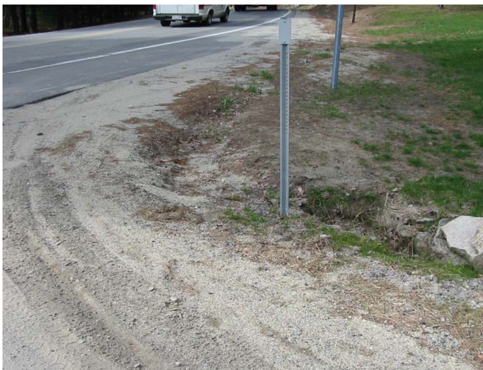
Figure 4-6 Sediment from Exposed Road Shoulder is Being Transported into Brook through Culvert
