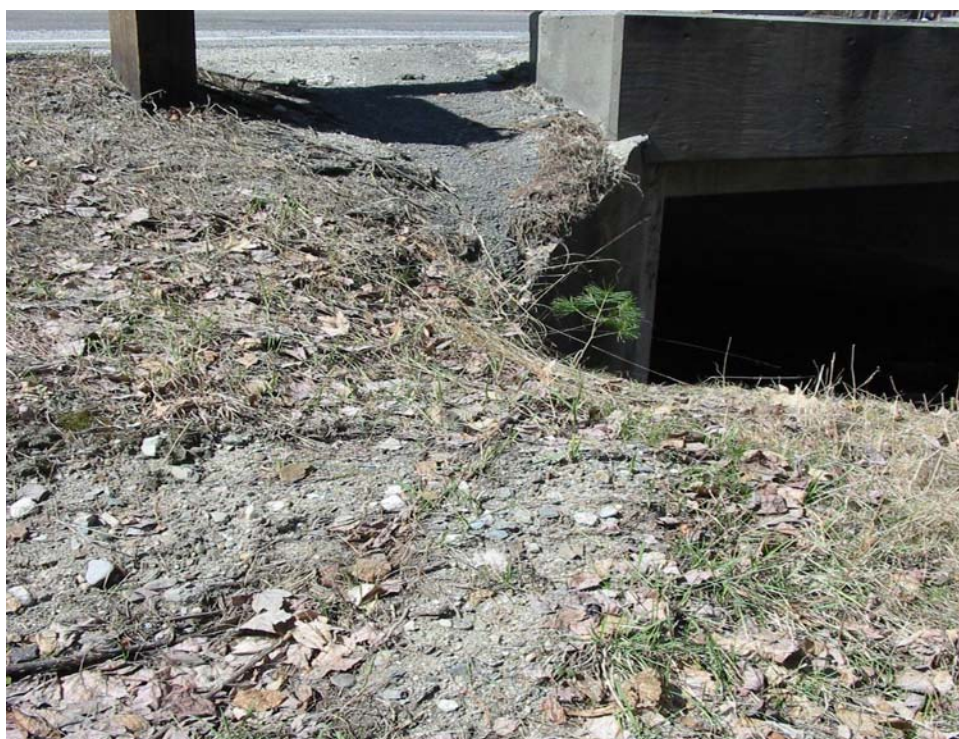
Figure 4-10 Sediment Trail and Paved Channel Leading into Culvert from Street Runoff
