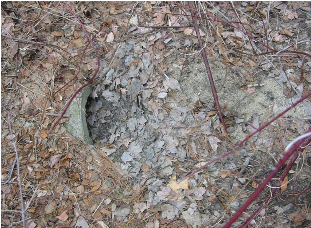
Figure 3-26 Clogged Outfall Pipe and Sediment Trail a Few Feet from the Brook from Ciro's Restaurant Parking Area Discharge
