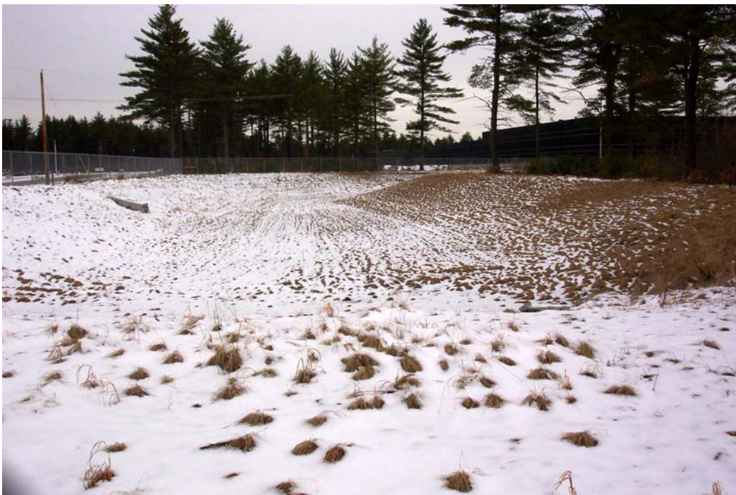
Figure 3-19 Large Detention Basin Captures Commercial Site Runoff for Recent Northwest Boulevard Development
