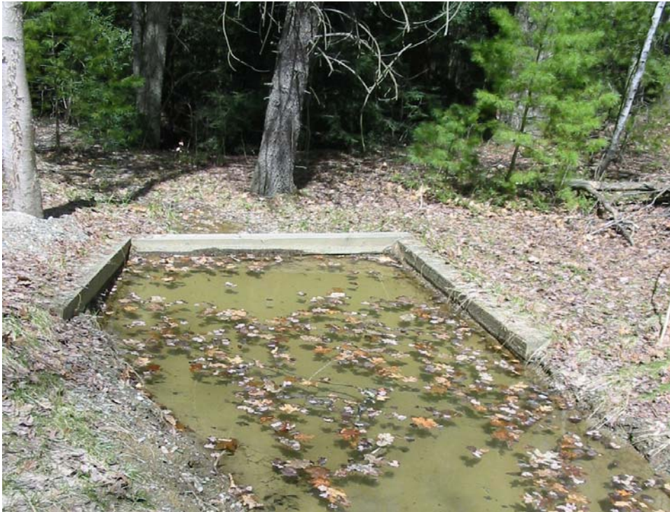
Figure 4-4 Working Sediment Trap with Ponded Stormwater
