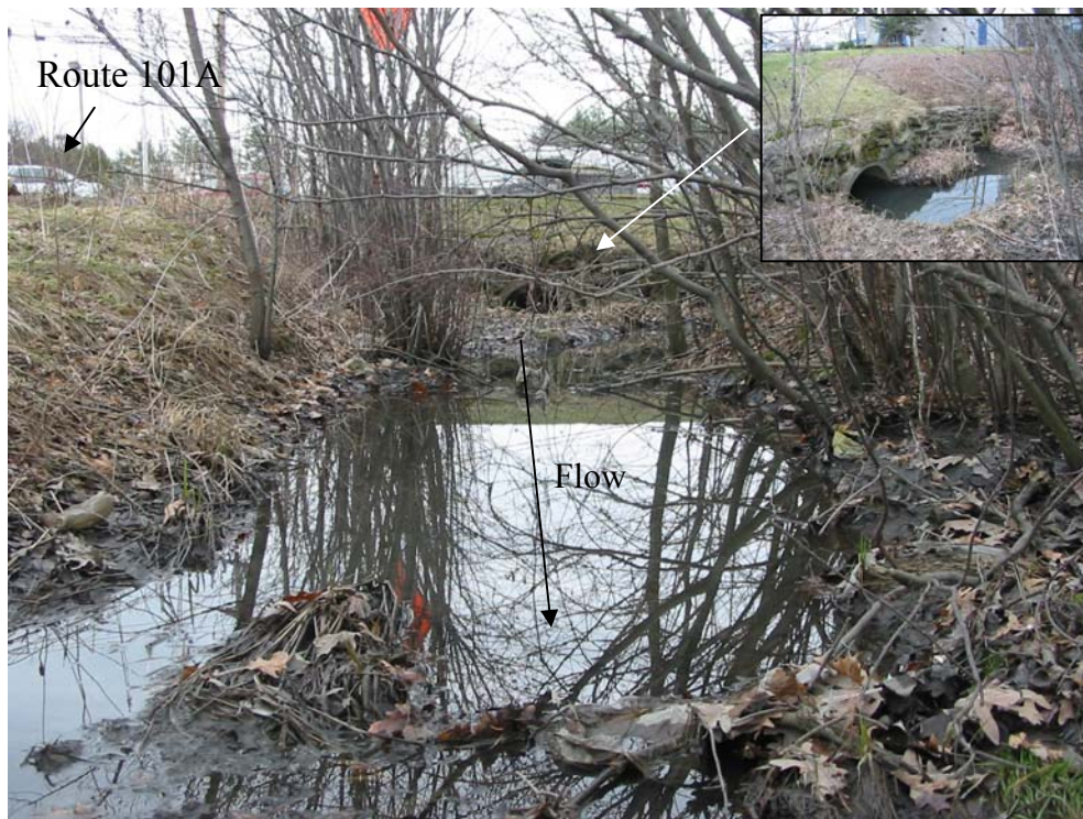
Figure 3-22 Channel Scouring from Route 101A and Greystone Plaza Stormwater Discharge Near Pennichuck Brook
