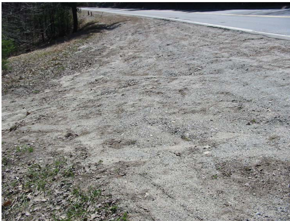
Figure 4-9 Exposed Dirt Shoulder Contributes to Sediment in Brook
