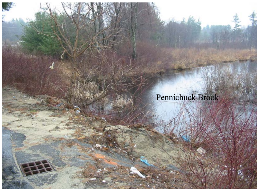
Figure 3-24 Clogged Catch Basin & Bank Erosion behind Pennichuck Square Plaza
