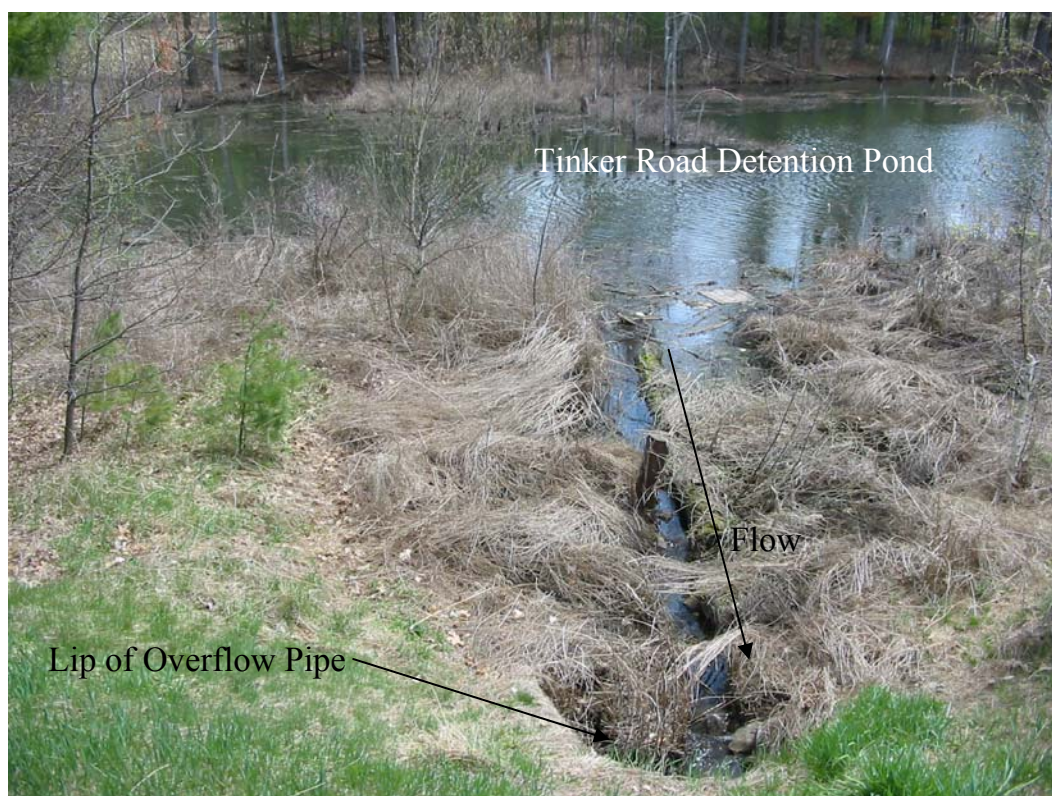
Figure 2-15 Overflow Channel Allows Untreated Stormwater to Enter Harris Pond
