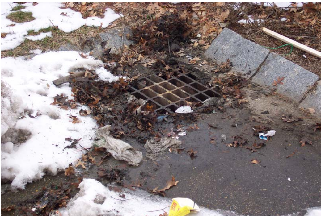
Figure 3-17 Trash and Debris Transported in and near Catch Basin from the Westside Plaza Parking Lot can Degrade Water Quality of Downstream Waterways
