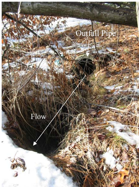
Figure 2-20 Channel Erosion Caused by Turnpike Bridge Discharge before Flowing into Bowers Pond
