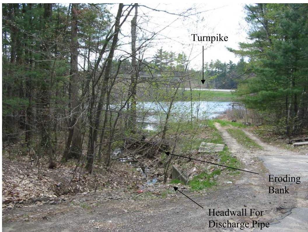
Figure 2-7 Eroded Bank and Strewn Debris at Tinker Road Detention Pond
