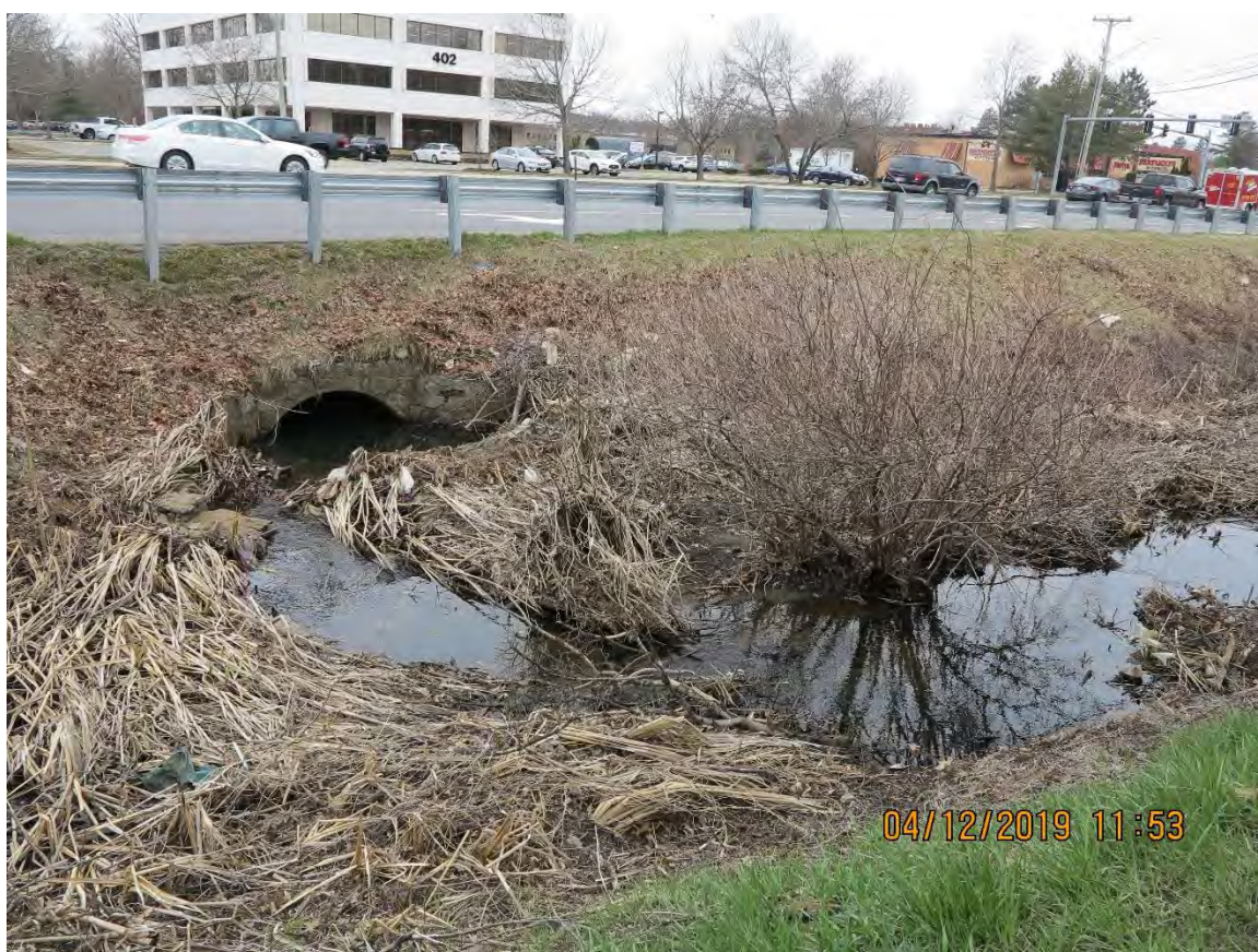
BMP SITE 4: Somerset Parkway Swales
