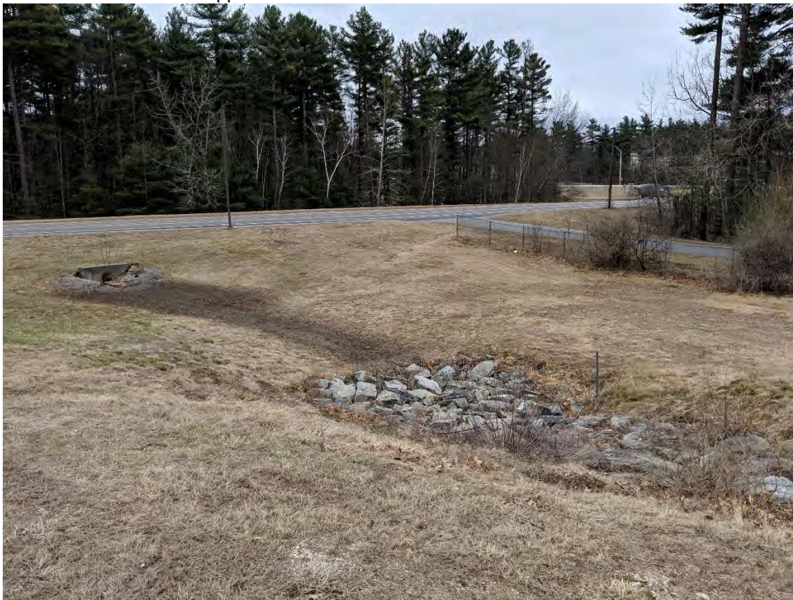
BMP SITE 8: Park & Ride Lot Detention Basin
