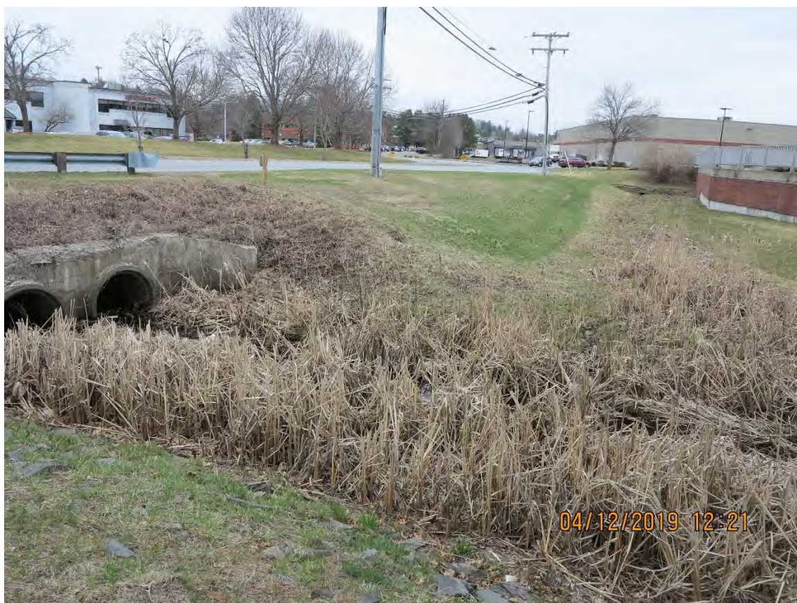
BMP SITE 4: Somerset Parkway Swales
