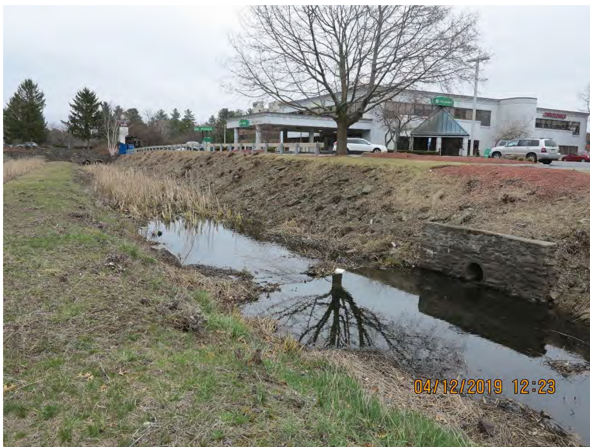
BMP SITE 4: Somerset Parkway Swales
