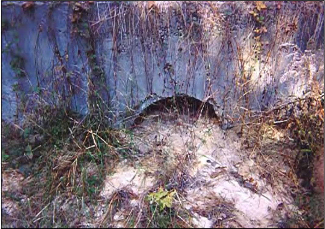
Figure 2-16. Cornerstone Discharge Blockage
