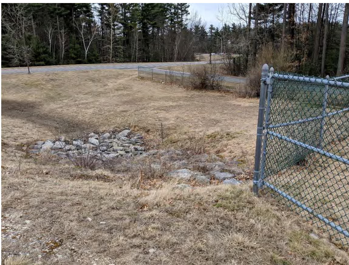
BMP SITE 8: Park & Ride Lot Detention Basin
