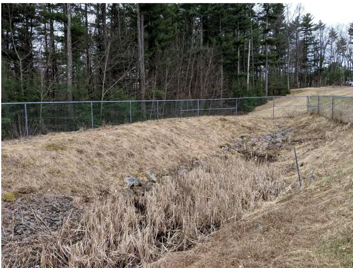
BMP SITE 8: Park & Ride Lot Detention Basin
