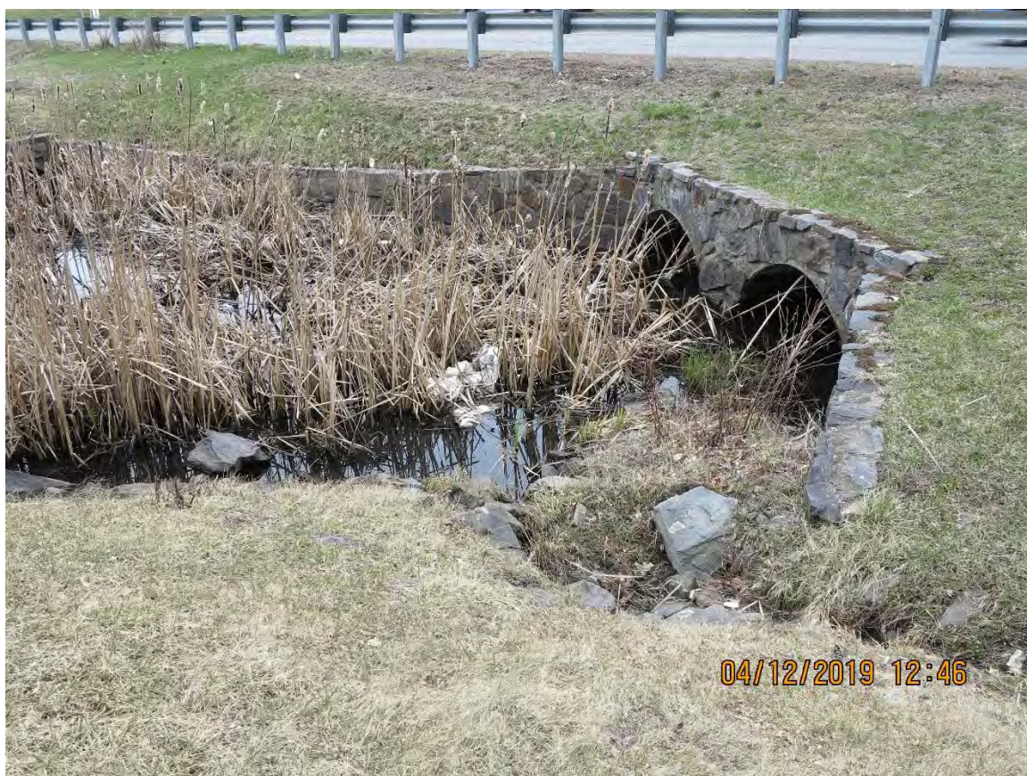
BMP SITE 4: Somerset Parkway Swales
